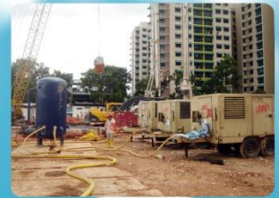
COMPRESSED AIR RESERVE
