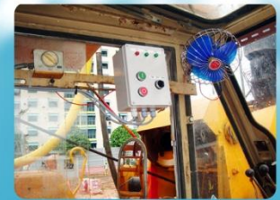
CONTROL BOX IN THE CABIN
