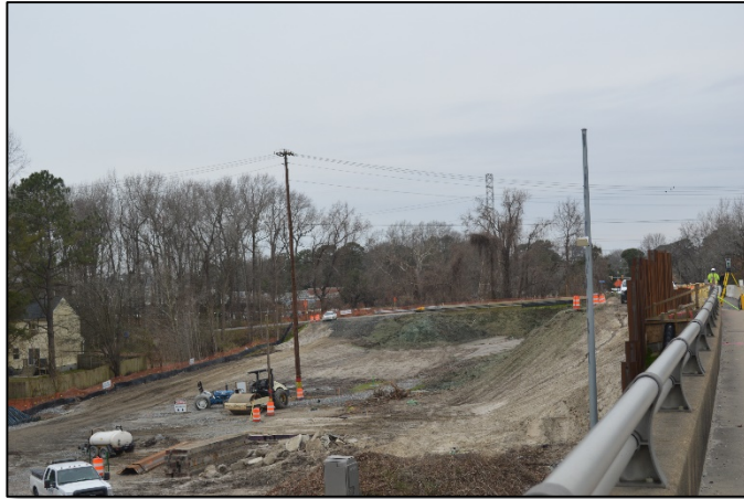
Crews prepare land for construction of the new Great Bridge Boulevard Bridge over I-64
