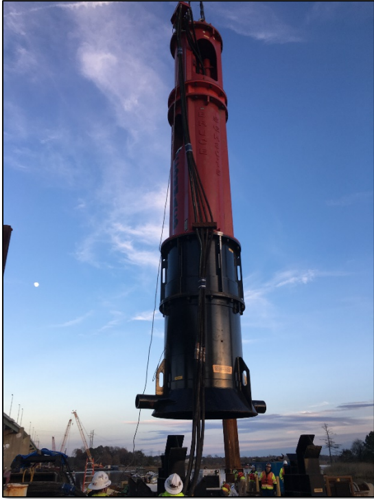
A Bruce SGH 3515 Hydraulic hammer is used in the 66" cylindrical pile-driving operation.
