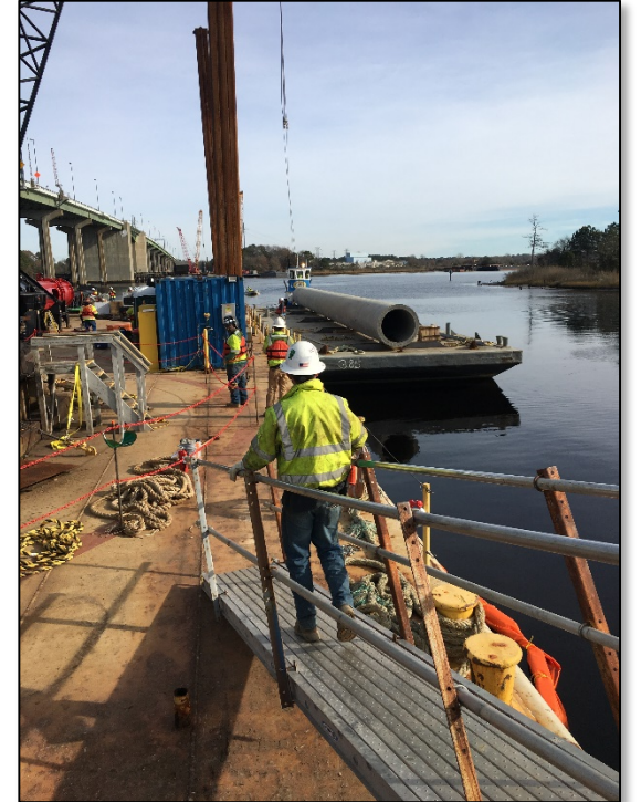
Crews prepare to begin the first test pile drive in the Elizabeth River. [Photo taken from east of the High Rise Bridge looking toward Virginia Beach.]
